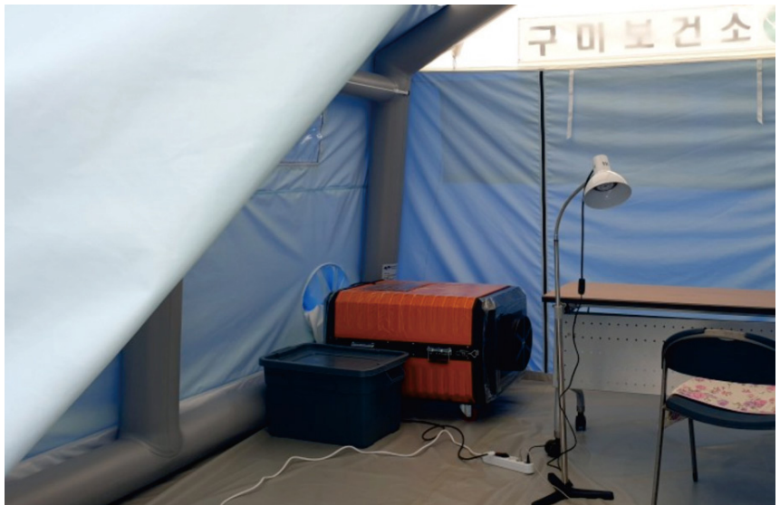
Installation completed in the negative pressure isolation tent of COVID-19 Screening Center
